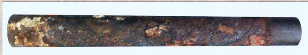
Figure 1: Pipe with Grease Tape after 10 Years
