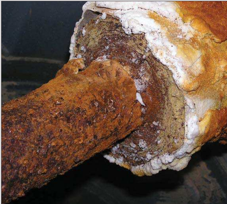
Figure 13: Pipe and Insulation after 2 years
