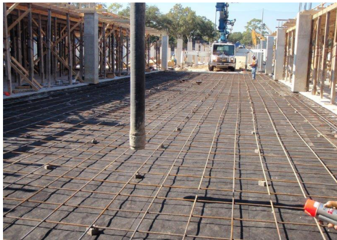
Polyguard Underslab in a center section of the floor prepared for concrete placement. Note the columns with pre-formed column boots.
