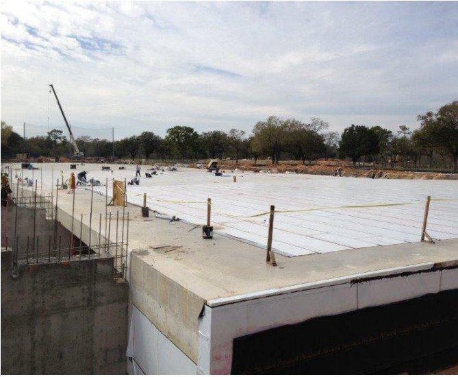
Under construction photo of the garage lid with the Polyguard 650 installed. Ramp tunnel to the left of the photo.
