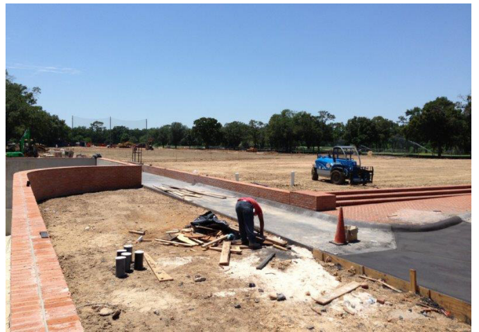
Completed garage and ramp areas covered with Poly Flow 18 drainage composite and backfill. The next step is sod installation.
