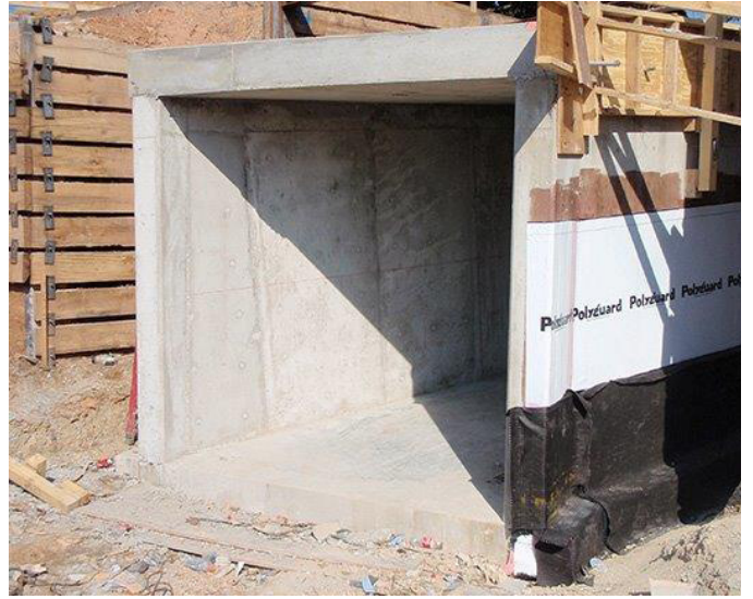
Section of the clubhouse tunnel with Polyguard Underslab beneath the slab and Polyguard 650 with Poly Flow 15P surrounding all sides. The Situra Flamline expansion joint connected the tunnel sections.
