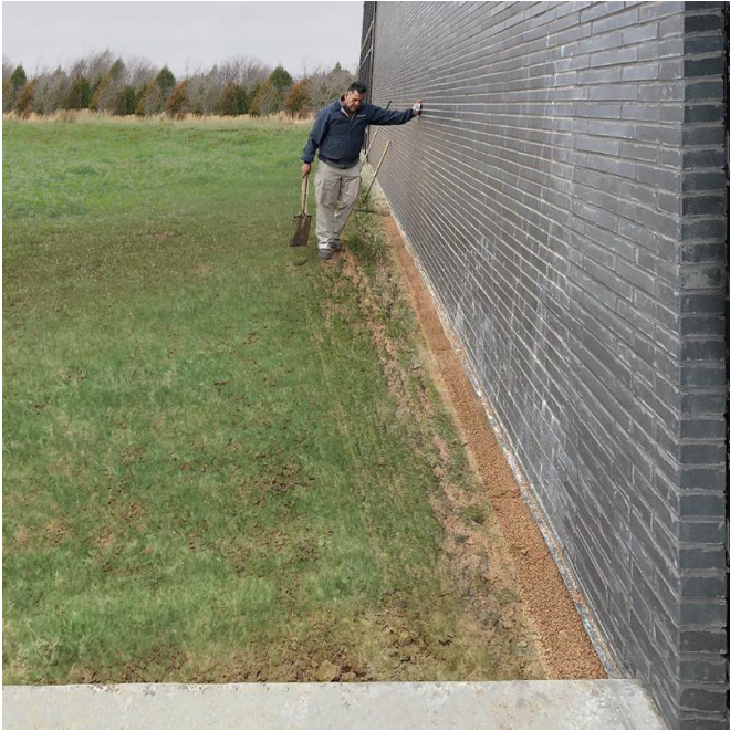
TERM Particle Barrier installed around exposed perimeter concrete at an Oklahoma hospital
